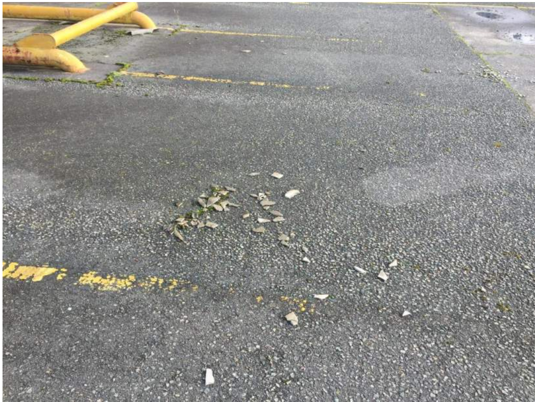
Photo 7: Potential loose asbestos on the hardstanding south of the warehouses.
